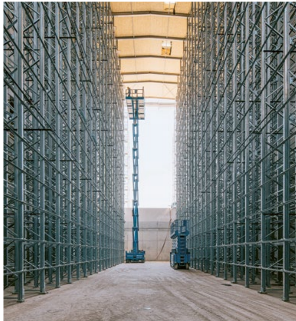
The new high-bay warehouse offers additional storage possibilities and optimises logistics as well as further processing of sawn timber.
